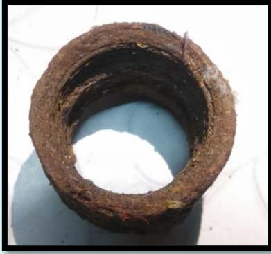
Corroded cast iron straight pipe joint
