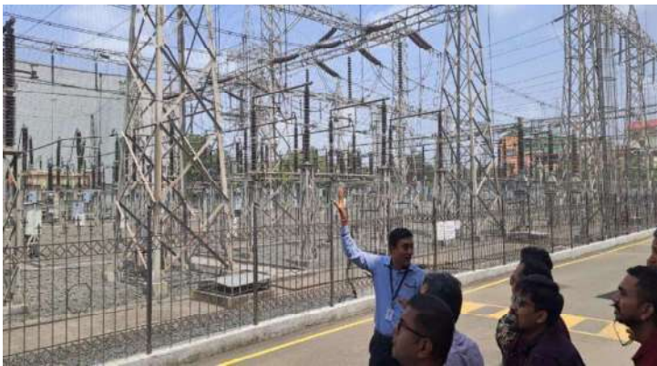
220 kV Gas Insulated Substation, Torrent Power, Surat
